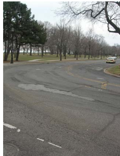
Sheridan Road through Evanston. This segment of roadway will be resurfaced with Recovery Act funds.
